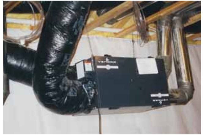
Figure 9. Heat recovery ventilators are seen in some new tightly constructed homes and added to existing tight homes.
