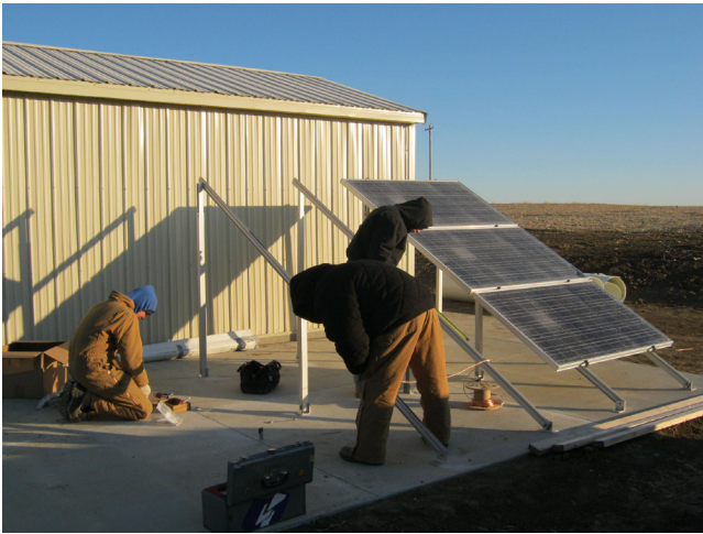
Figure 2. Installation of a solar PV system requires careful preparation to ensure a safe, long-lasting operation. This solar array is installed near Concord, Nebraska. For live data from this solar array, visit http://bioenergy.unl.edu .
