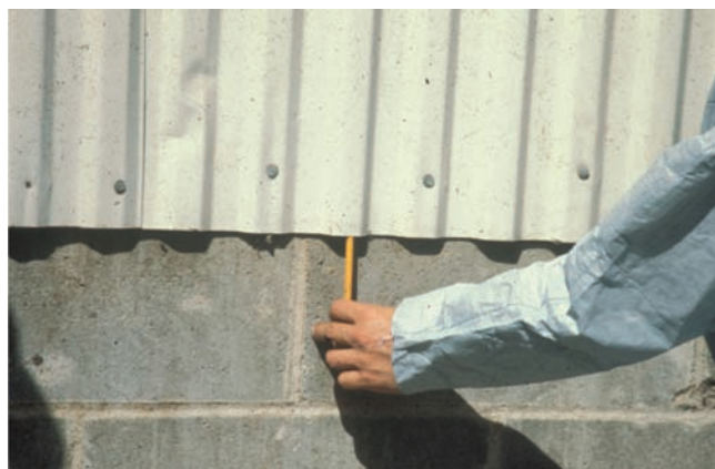
Figure 3. Mice can enter the wall space where the ends of metal siding panels are open by gnawing through the weather shield or vinyl gasket. Use concrete, angle iron, or heavy duty flashing to block access to rodents. Photo by Rex O. Baker.
