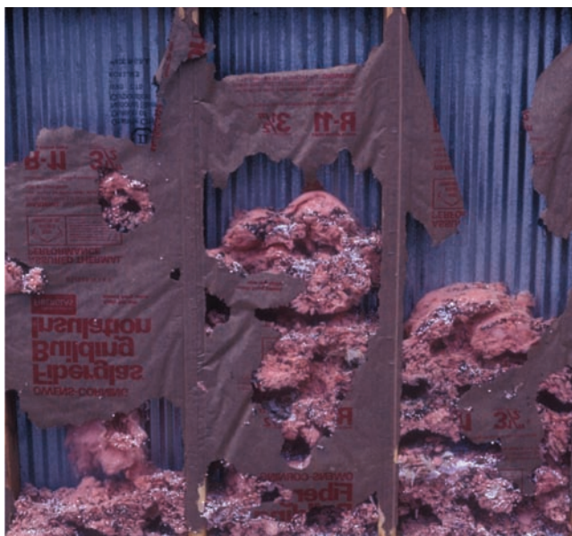
Figure 1. Mice can quickly destroy insulation in walls. Damage this extensive can occur in as little as three years. Photo by Robert M. Timm.
