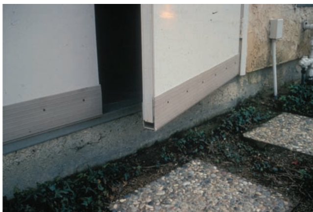
Figure 5. Metal flashing or a metal channel prevents rodents from gnawing at the bottom edge of a door. Photo by University of Nebraska–Lincoln Extension.
